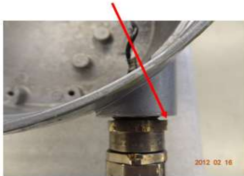
Figure 13: Gap between gland and the VITO housing - not allowed
